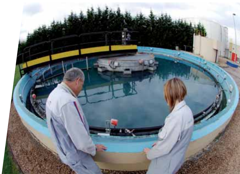
Trémery plant (France), ultra-filtration unit.
