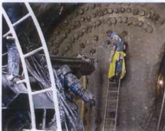
Horizontal jet grouting injection of a bulkhead. The yellow pipe at the drilling mouth is connected to the 'preventer'
