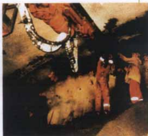
Figure 11 (above): Installation of a grouted pipe umbrella (screen) in the Irlahüll tunnel
