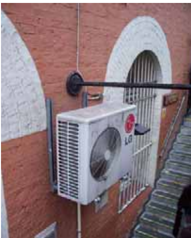
Figure 103: External air conditioning equipment at ground floor level. St Vincent Centre, Carlisle Place
