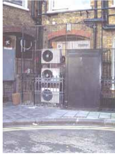
Figure 104: air conditioning units on King Scholars Passage
