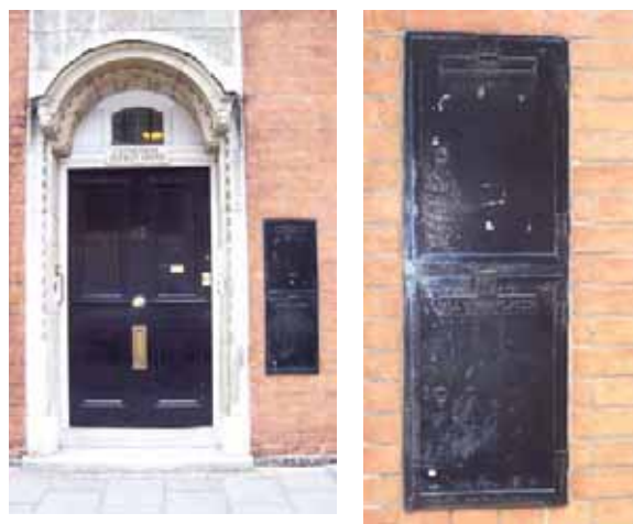
Figure 85 & 86: Decommissioned wall mounted letter boxes (Clergy House, Francis Street)
