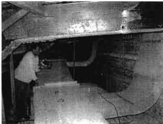
Figure 2 – Existing extract duct indicates space available under upper circle
