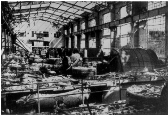
Figure 1. Destroyed Lardarello No 2 Station Turbine Hall.
