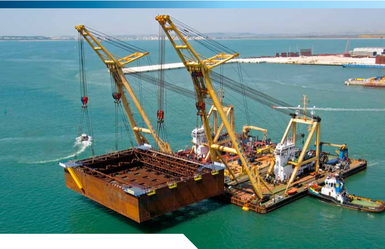
SMIT Heavy Lift installed the caissons for a new bridge in Cadiz.
