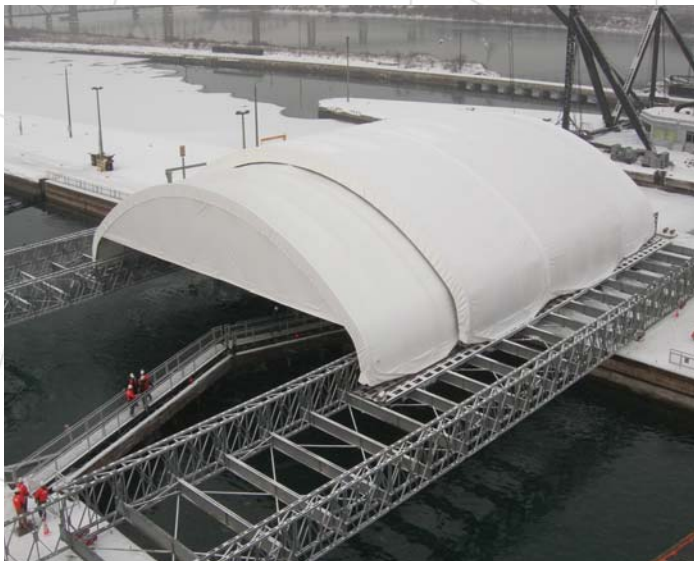
Critical repairs and upgrades that are part of the Asset Renewal Plan must be completed during the short 10-week period that the Soo Locks are shut down each winter.
