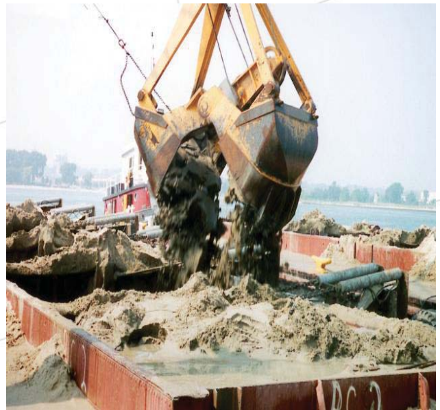
Hydraulic dredging (top) and mechanical dredging (above) are the types of dredging operations used to clear channels and harbors on the Great Lakes.
