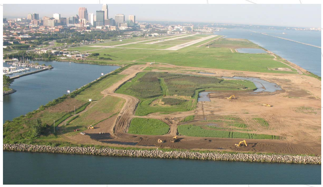
Dredging at Cleveland Harbor is currently limited by disposal capacity. Interim measures to increase capacity are being employed while construction of a new CDF is being planned.
