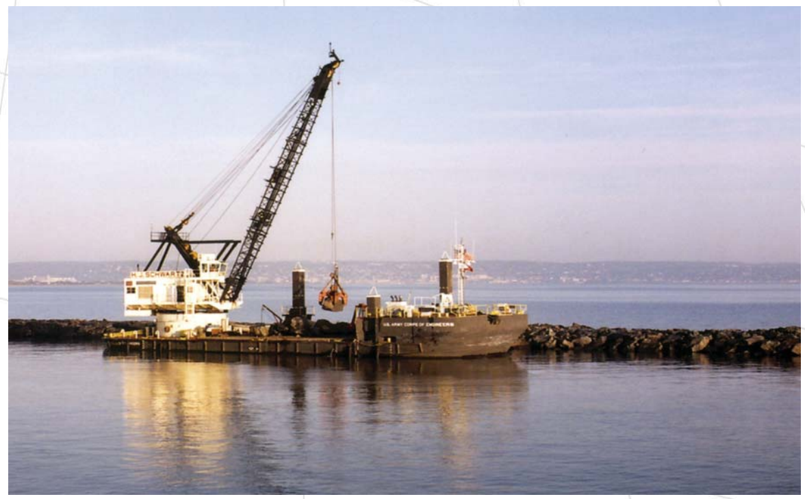
The Corps floating plant performs maintenance and emergency repairs at breakwaters across the Great Lakes.
