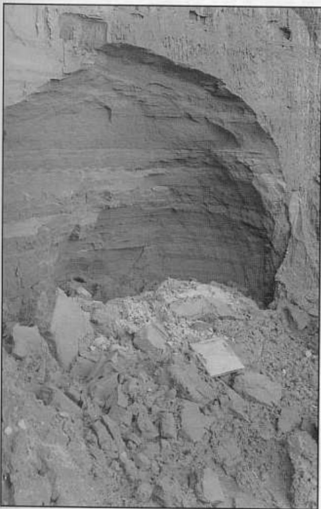
Figure 43. Seepage erosion in glaciofluvial sand at gravel pit in Coquitlam River valley. Note field book for scale (courtesy of O. Hung, Thurber Engineering).
