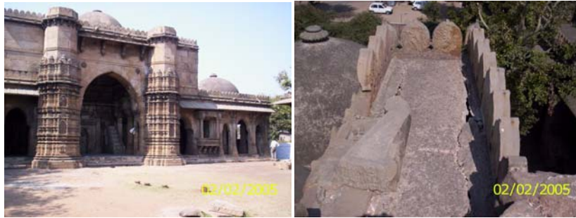
Figure A.1 – Geometry: (a) front view of Tomb (b) distressed walls of Tomb
