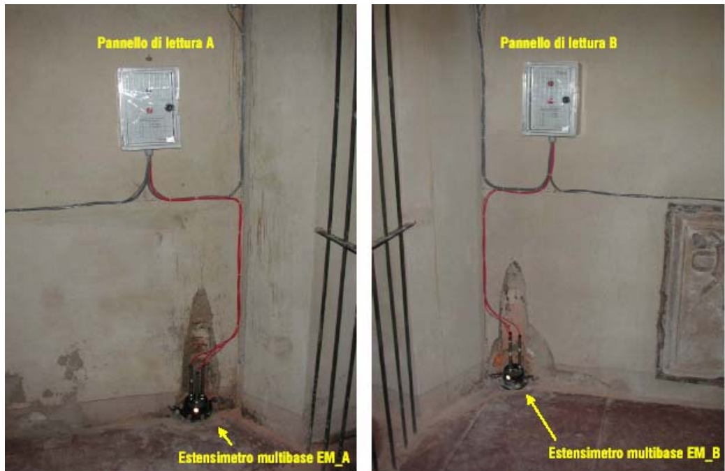
Figure 20: measurement panels A and B and view of the top of the multi-base extensometers
