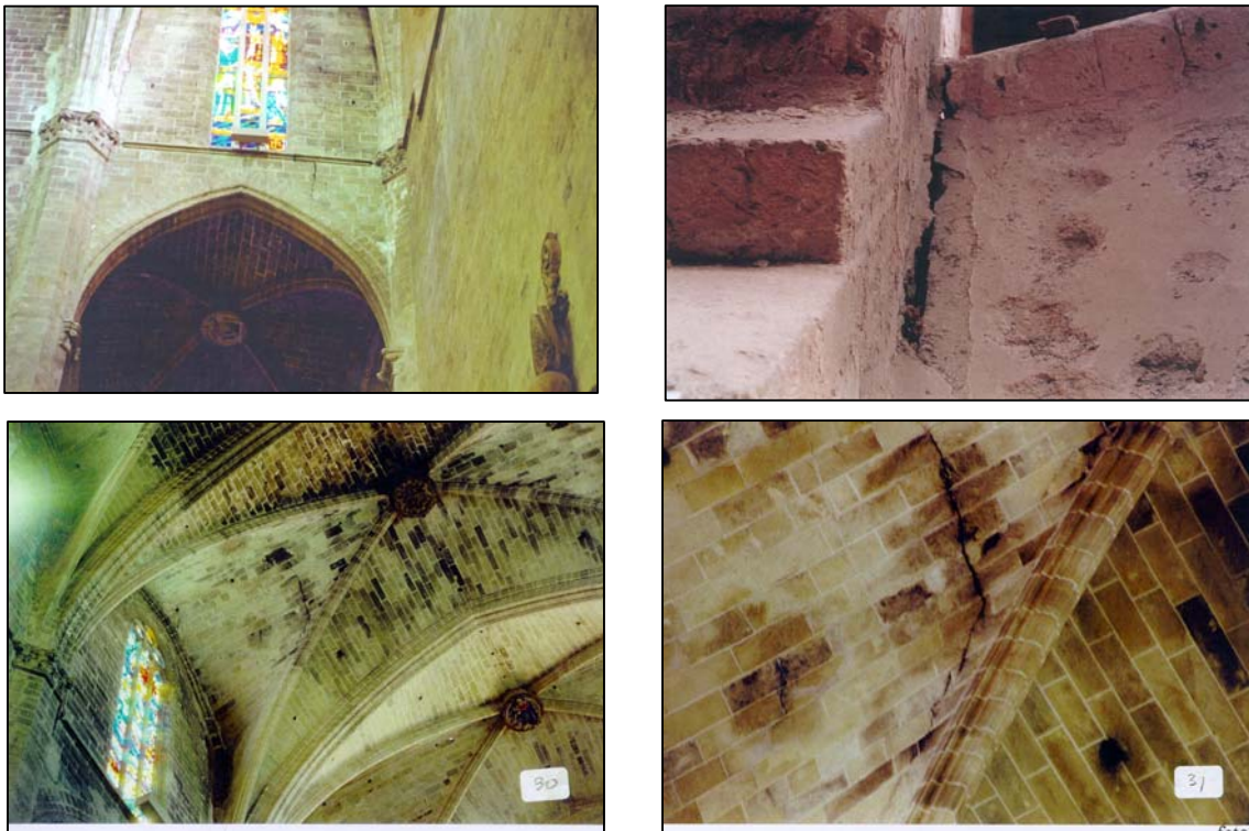
Figure 13 – Examples of cracking in (left, above) the clerestory, (right, above) between vault and transverse arch and (below) in the vaults of the central
