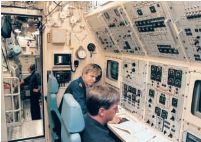
An advanced control and supervisory system is used for both the AIP unit and the conventional electric motors and diesel engines.
