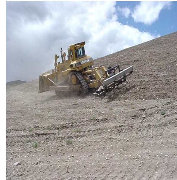
Seeding of the slopes of the heap leach pile, after side tracking and roughening.
