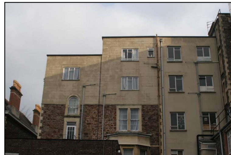
Poor quality extensions and infill jar with the historic fabric of the buildings
