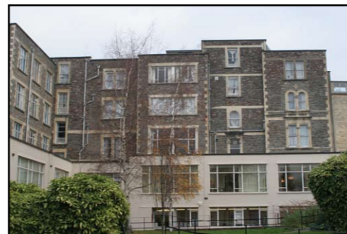
South elevation has lost rhythm through changed window openings from vertical to horizontal emphasis
