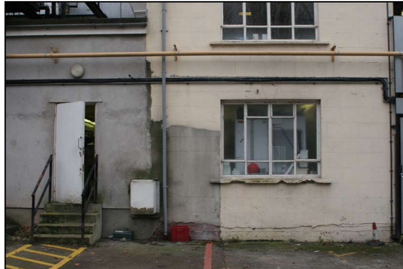
1950s materials decaying badly
