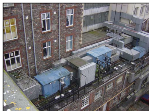
Plant room on rear kitchen extension
