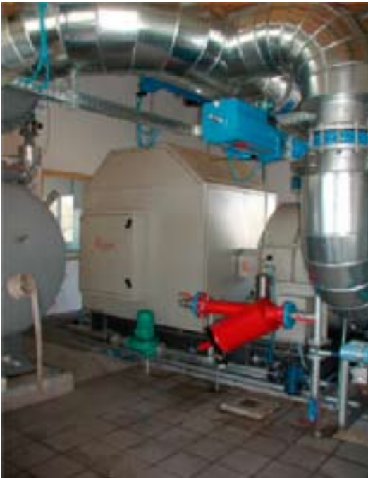
Figure 3: Altheim Binary Plant.
