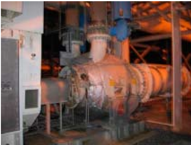
Figure 14: Salavatli Binary Plant.
