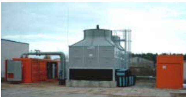
Figure 6: Neustadt Glewe Binary Plant.
