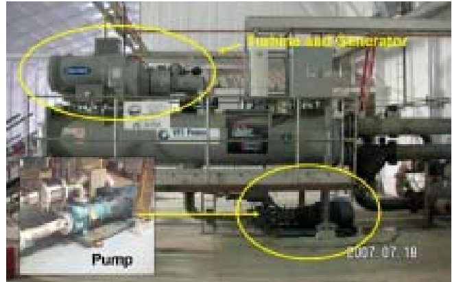
Figure 15: Chena Binary Plant.
