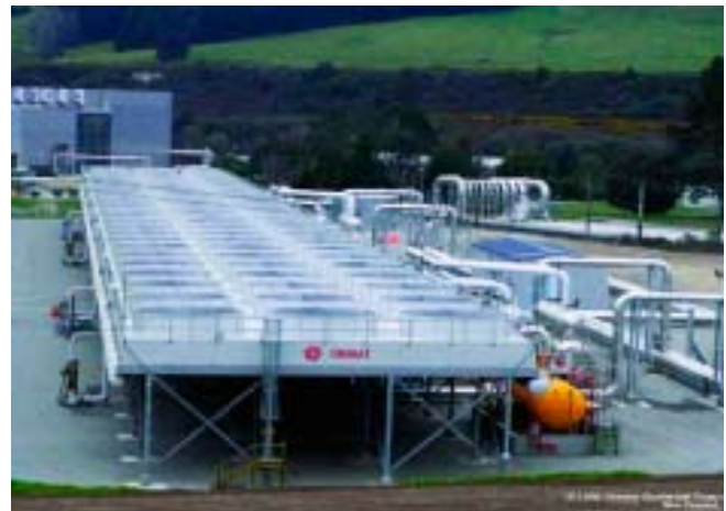
Figure 9: Wairakei Binary Plant.
