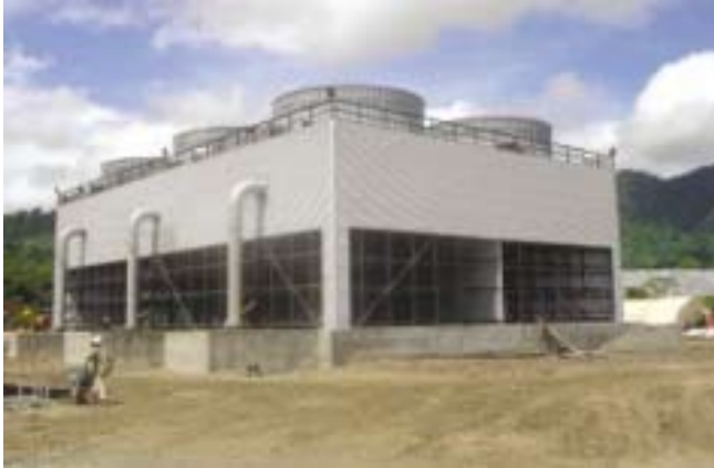
Figure 10: Lihir Back-Pressure Steam Power Station.
