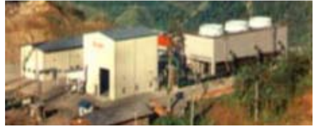
Figure 11: Leyte Binary Plant.
