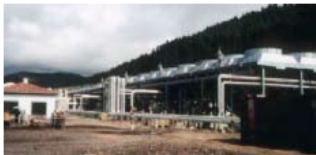
Figure 12: Ribeira Grande Binary Plant.
