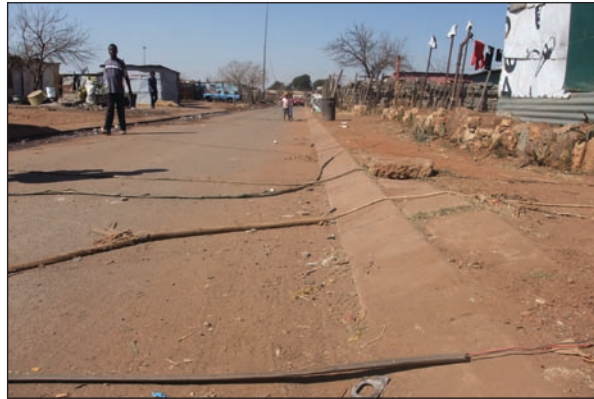
Illegal electricity connections in Thokoza
