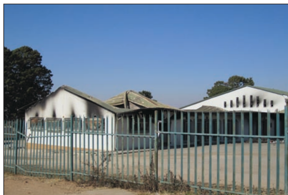
Burnt-out community hall in Thandakukhanya
