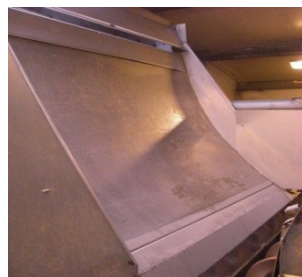
Picture 2: Internal side of the filter.
