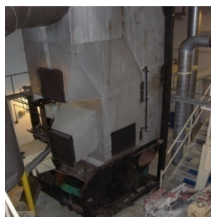
Picture 1: Crusher + ventilator
