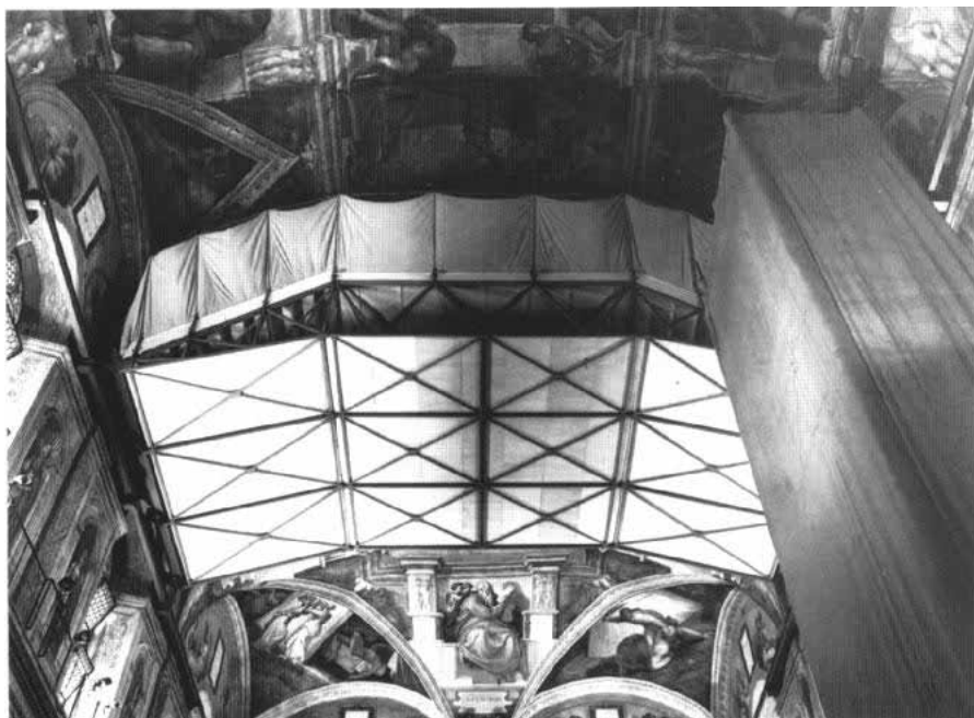
Figure 3. View of the mobile scaffolding used for the conservation, with the access tower shown at right.
