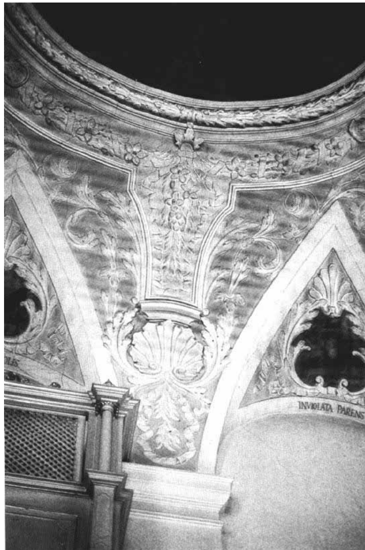
Figure 6. Damage resulting from the different thermal conductivity of plaster and wooden lath.
