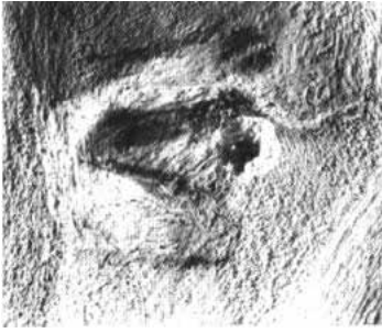
Figure 5. A funnel-shaped loss in the render caused by the slaking of calcium oxide. Photographed in raking light. 1984.
