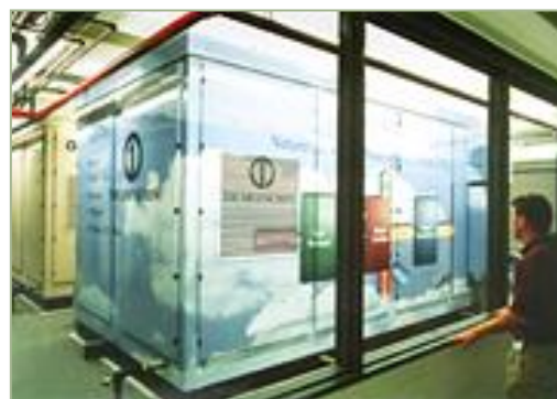
First National Bank of Omaha's fuel cells provide high quality, reliable power to their data processing facility
