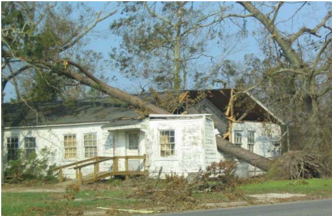
Picture 2. Example of damage in Orange County, TX caused by Hurricane Rita. Photo taken by WFO Lake Charles, LA.
