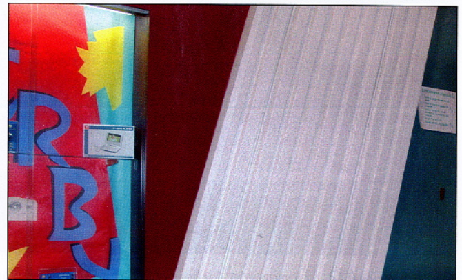
On this cafeteria wall at Woodward Middle School (Bainbridge Island, Washington), perforated metal provides not only protection for other sound-absorbing surfaces, but also acoustic improvement of its own.
