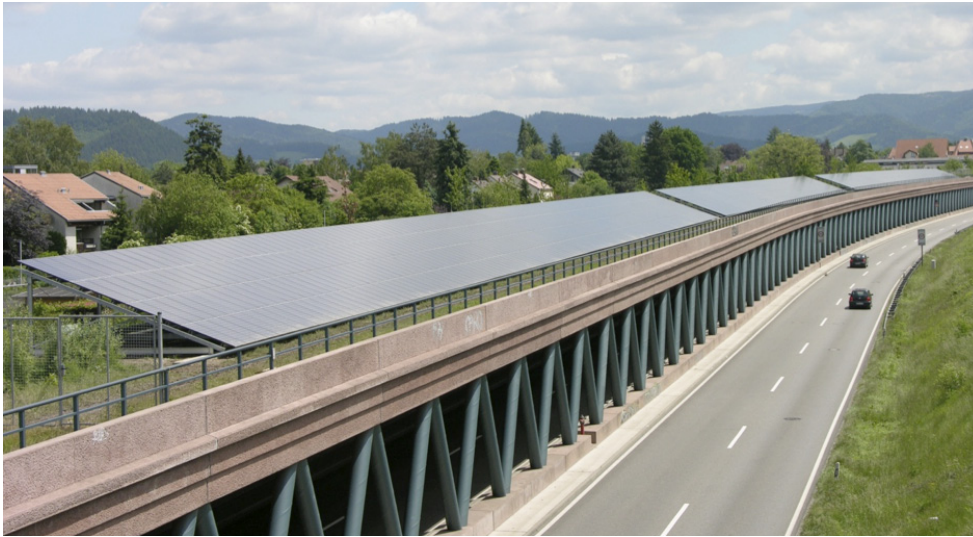
A community-owned PV array on a noise barrier in Freiburg, Germany. Source: fesa GmbH 2006
