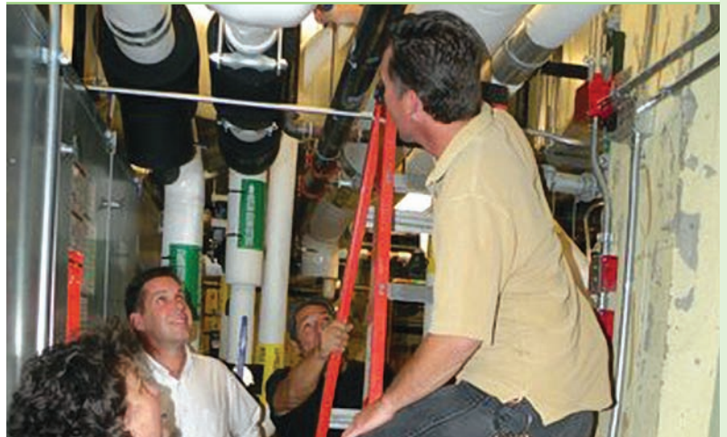
▲ Planet Blue Teams inspect HVAC systems in Rackham Building.
