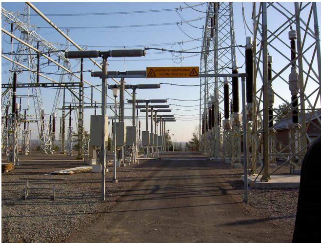
Fig. 1. DCB in Lindome 400 kV substation
