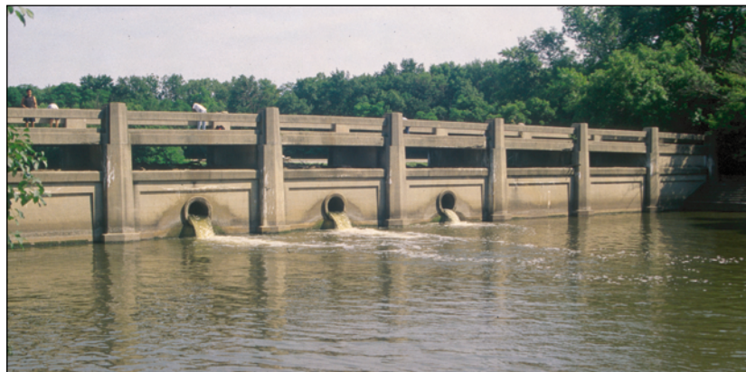
Willow Road Dam at the south end of Skokie Lagoons is the main control dam for the lagoon system (June 2004; photo by M. Chrzastowski, ISGS).
