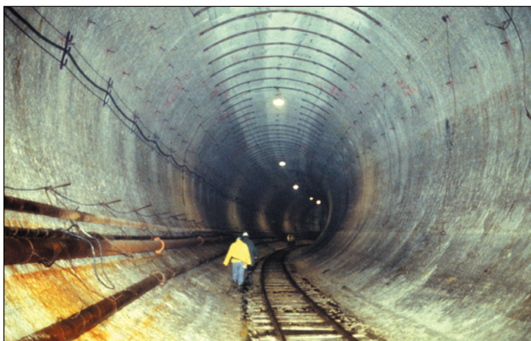
A person provides scale within an unlined tunnel segment in Silurian dolomite. This photo is from a tunnel system similar to TARP being built in Milwaukee County, Wisconsin (photo by Robert Bauer, ISGS).
