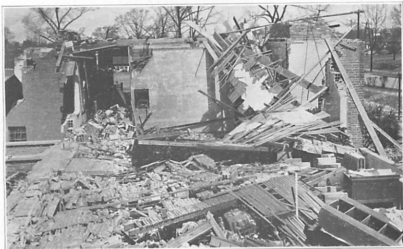
Figure 11.—A part of the west wall of the front section of the Church Street Grammar School was blown eastward across the small desks of that section by the tornado of April 5, 1936.--Photographed April 13, 1936.
