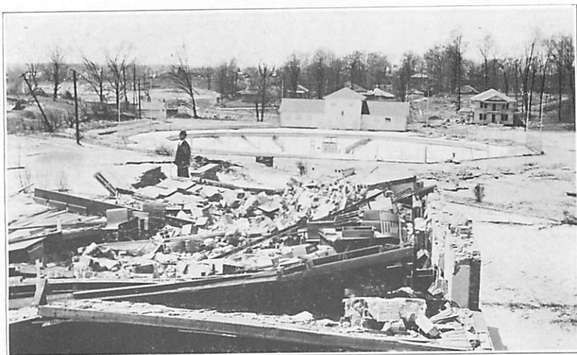
Figure 10.—The north wall of the north wing of the Church Street Grammar School was likewise blown southward across the small desks of that wing by the tornado of April 5, 1936.--Photographed April 13, 1936.
