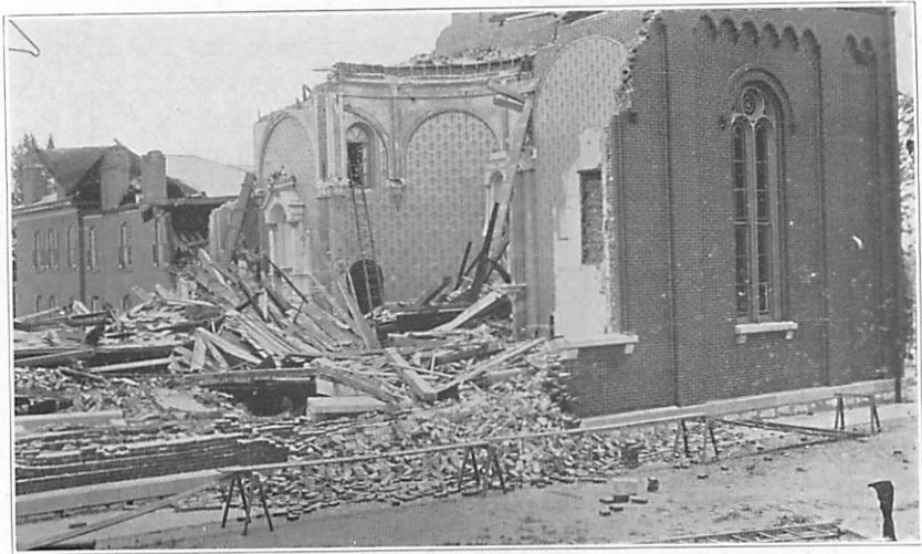
Figure 8.—Even frail partitions of the altar end of Borromeo Church, St. Charles, Mo., held the walls against the onslaught of the tornado of July 7, 1915. -- Photographed July 9, 1915.
