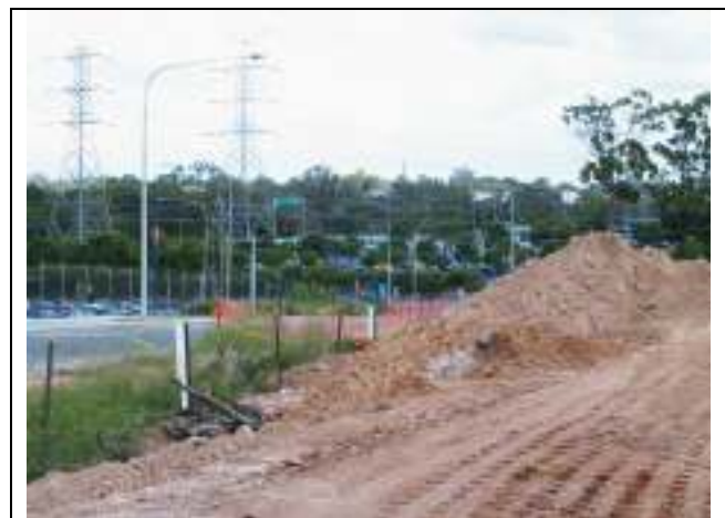
Centrus construction site with the Eight Mile Plains busway station and park and ride in the background
