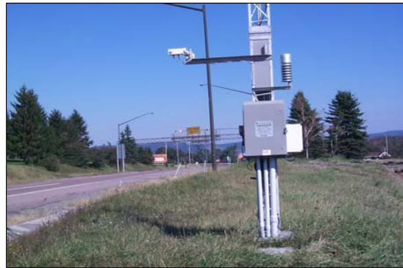
F Figure 8. Keysers Ridge RWIS station.
