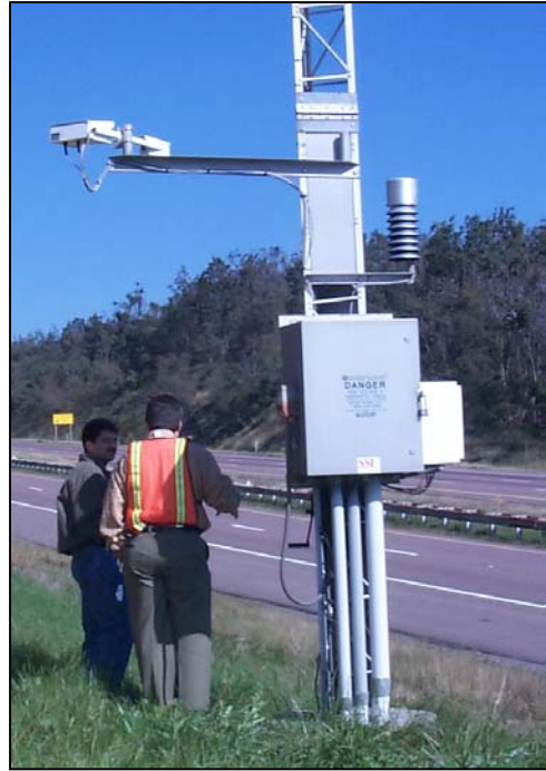
Figure 3. I-68 RWIS Station Located Near Big Savage Mountain.
