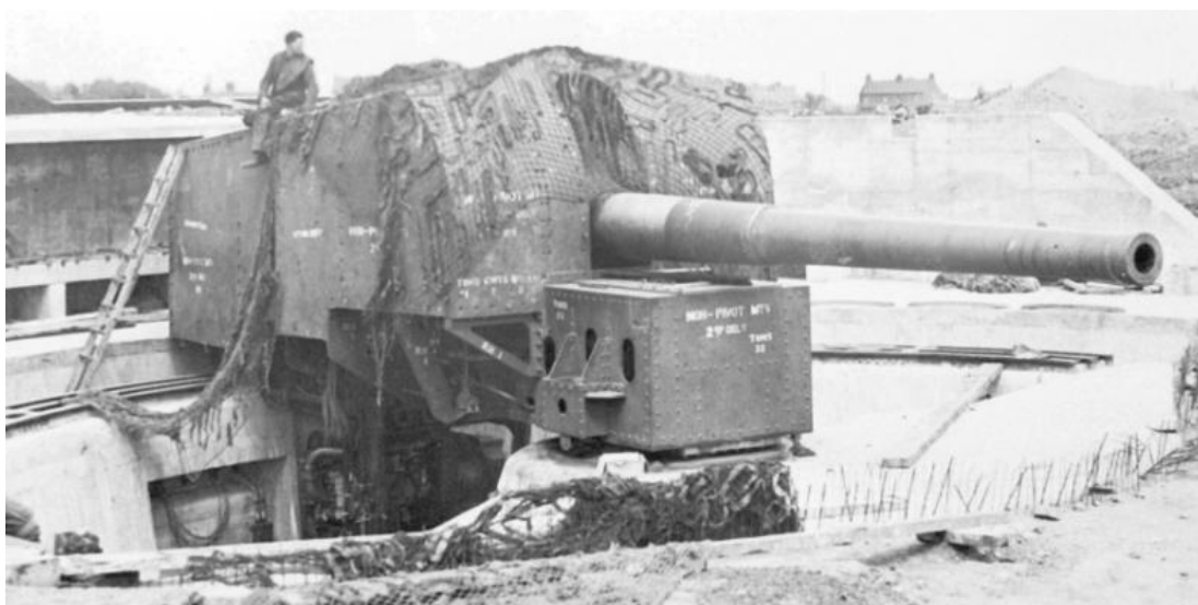
One of the gun installations for an 8-inch Mark 8** gun nearing completion at the Capel Battery near Folkestone during 1942
