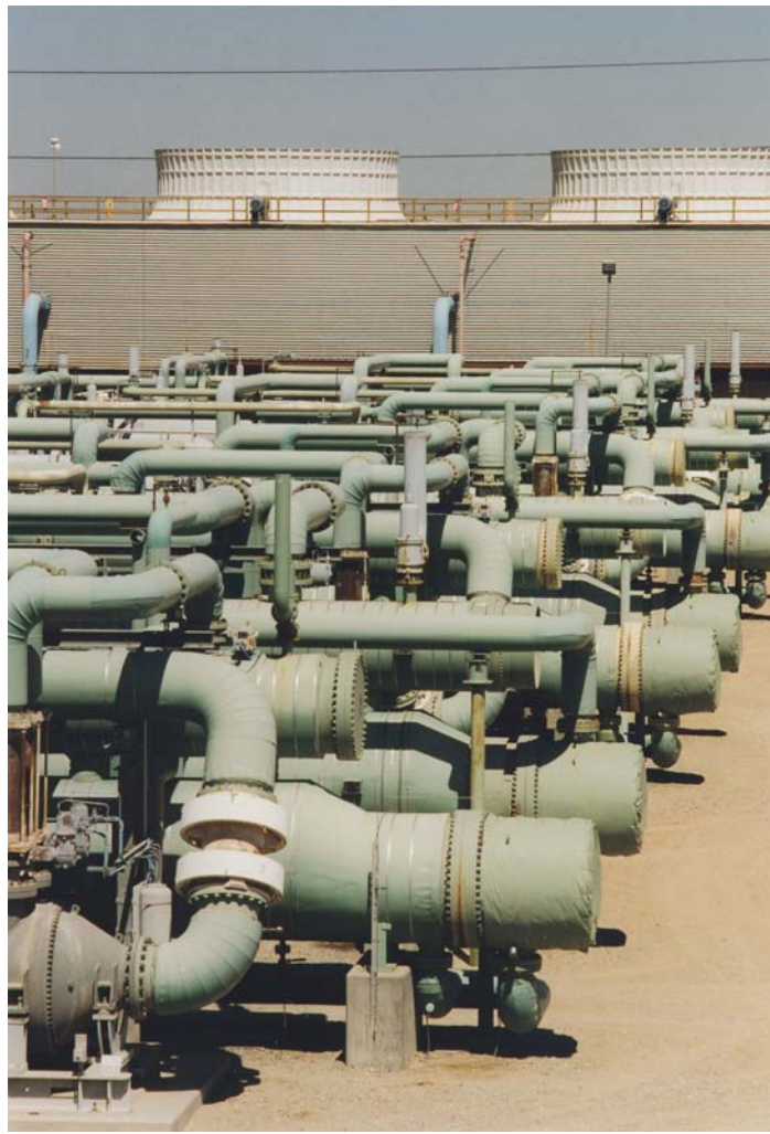
Planned improvements by East Mesa projects buyer ORMAT Nevada, Inc. will enable the projects to produce 25 percent more electricity for the California power grid.
