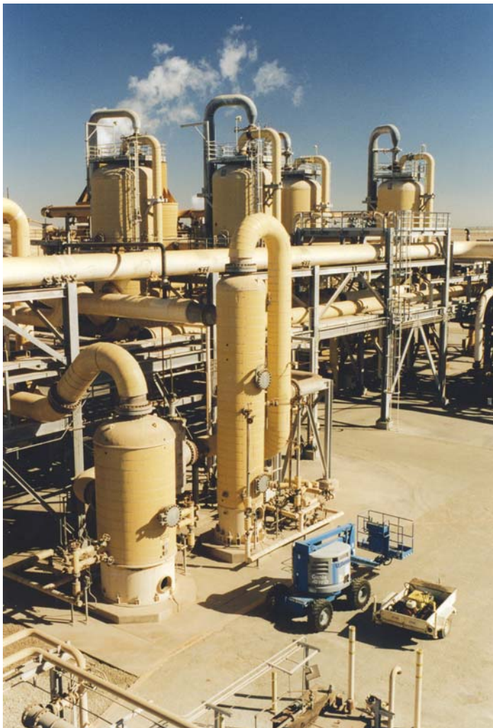
CalEnergy Operating Corp. currently produces over 340 megawatts from their geothermal power units 1 through 5 near the southern shores of California's Salton Sea.
