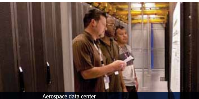
Aerospace data center
