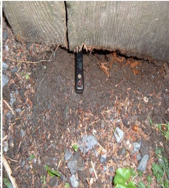
Extensive deterioration at base of pole
