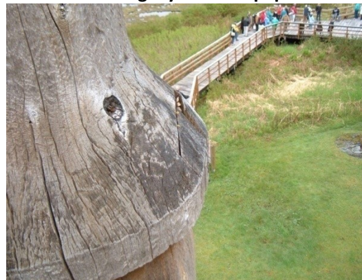
Repair patch that is loose
