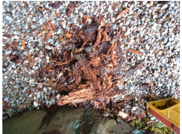
Decayed wood removed from behind knot
