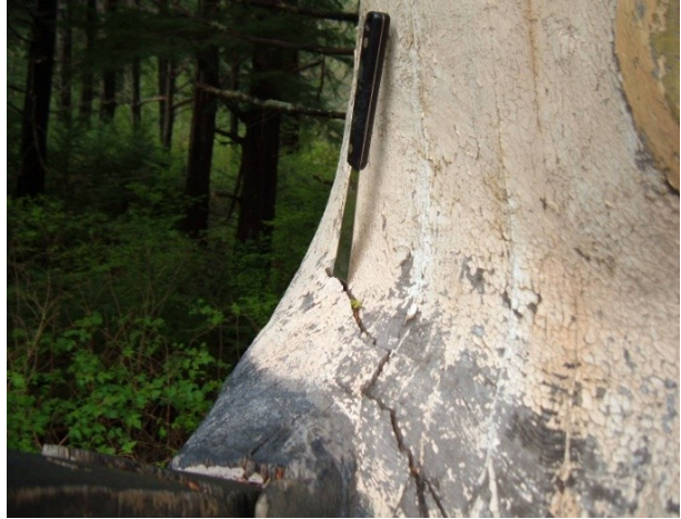
Separation at right shoulder
