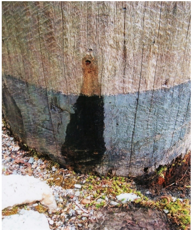
Water running out of knot hole
