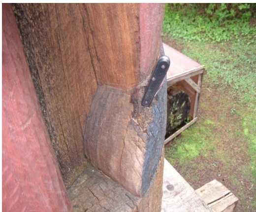
Deterioration in left foot
