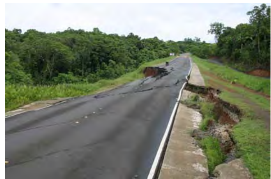
Figure 7 Collapsed national highway in Ngchesar State after heavy rains in 2009
