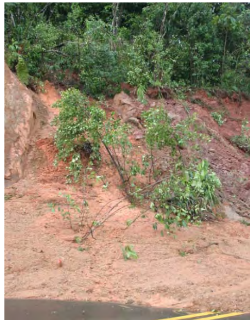
Figure 6 Chronic failure of slope along Compact Road at Ngaremlengui in 2009
