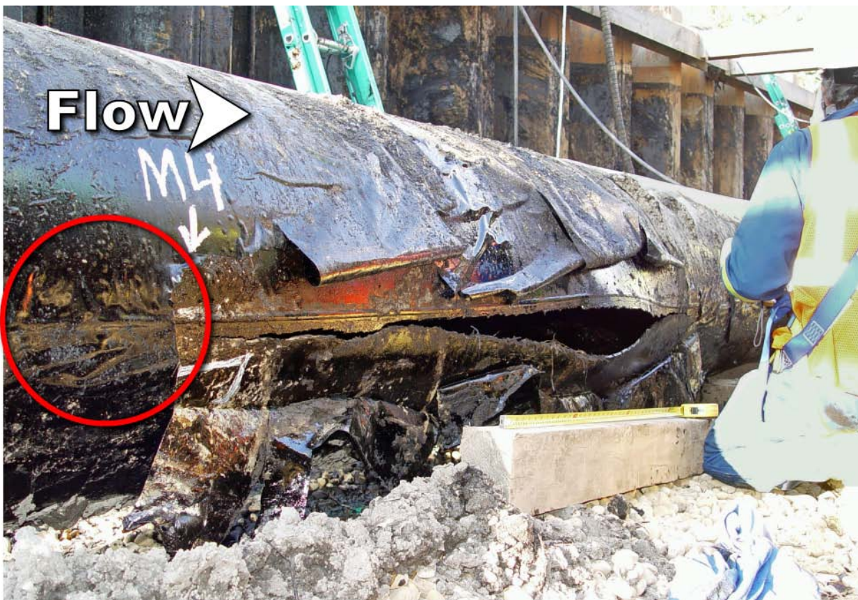
Figure 2. The ruptured segment of Line 6B in the trench following the July 25, 2010, rupture. The fracture face measured about 6 feet 8.25 inches long and was 5.32 inches wide at the widest opening. The fracture ran just below the seam weld that was oriented just below the 3 o'clock position. A red circle shows a location where the coating was wrinkled and had separated from the pipe surface.
