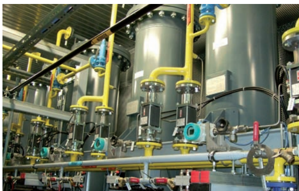
Photo 6. Upgrading plant, Malmö Sweden, using the PSA technology of Carbotech
