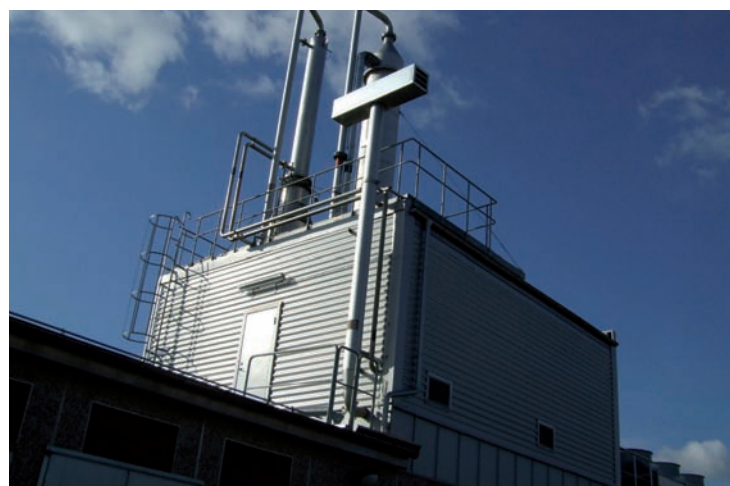
Photo 8. Upgrading plant in Gothenburg, Sweden, using the chemical scrubber technology. To the left the stripper column where the amine solution is regenerated by heat and to the right the absorption column.
