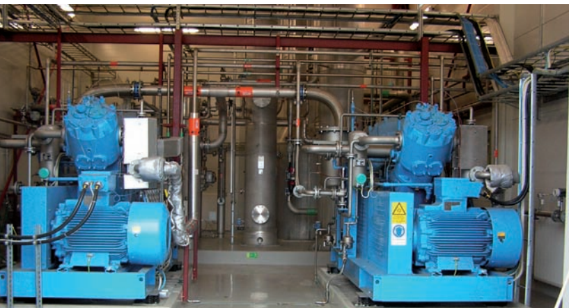
Photo 7. Kristianstad, Sweden, upgrading plant with a water scrubber. In the back the absorption column, flash tank and desorption column can be seen.
