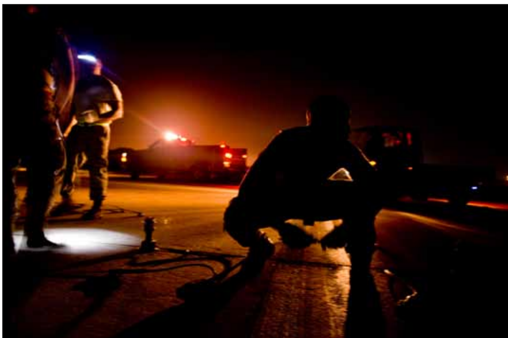
Airmen from the 8th Civil Engineer Squadron make final connections on an expeditionary runway lighting system at Kunsan Air Base, Republic of Korea, Sept. 30, 2013. The 8th CES took advantage of a break in the flying schedule to inspect a system not fully tested here in more than seven years. This system ensures the Wolf Pack can operate around the clock, even during a power outage. (U.S. Air Force photos/Senior Airman Armando A. Schwier-Morales)
