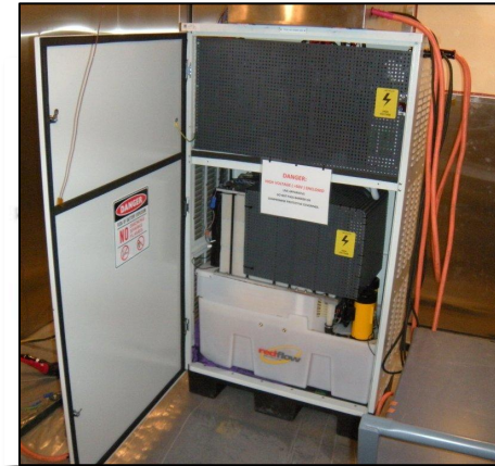
RedFlow 10kWh Zn-Br flow battery module and system (D. Rose)
