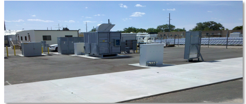
Energy Storage Test Pad (ESTP)
