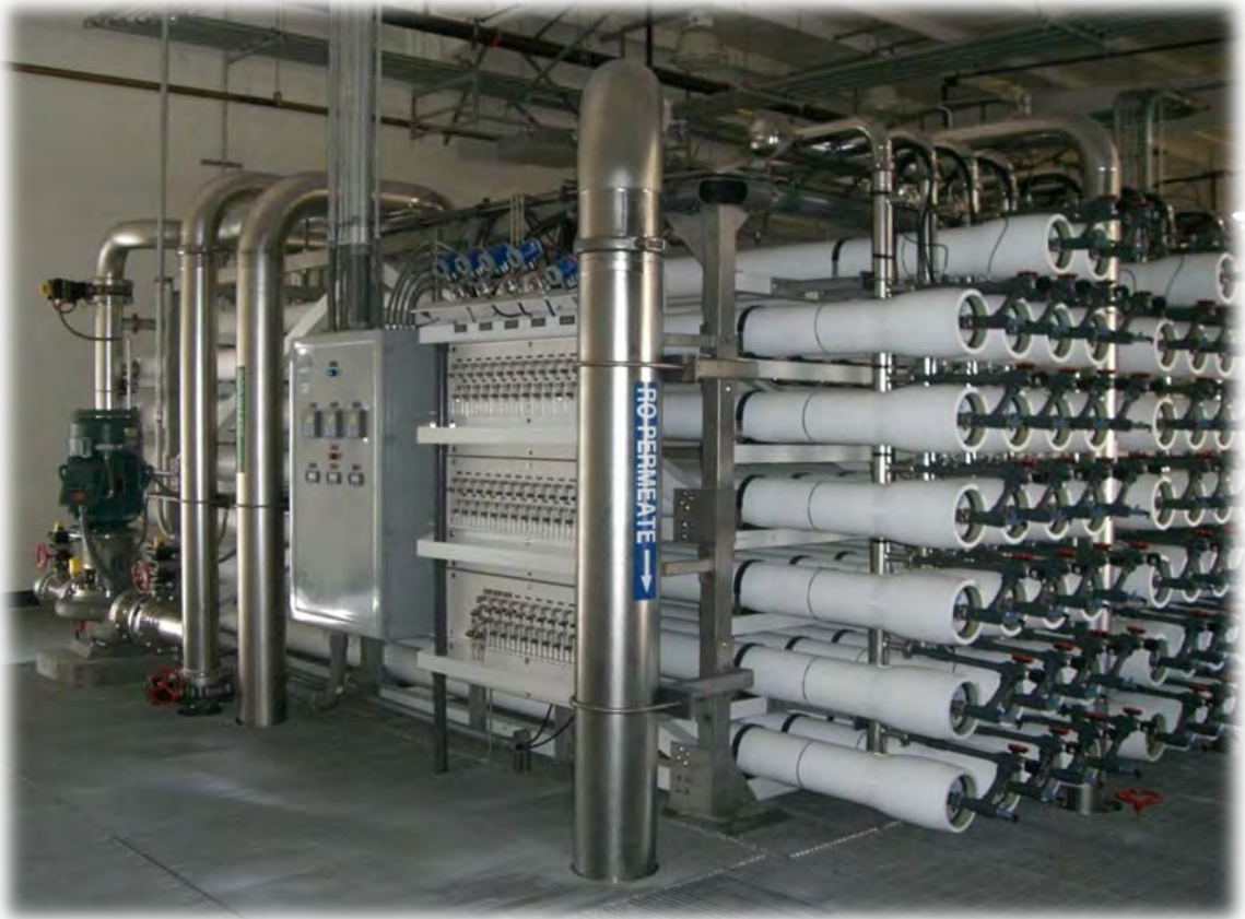
Figure 4.9 Two Stage Brackish RO Train
