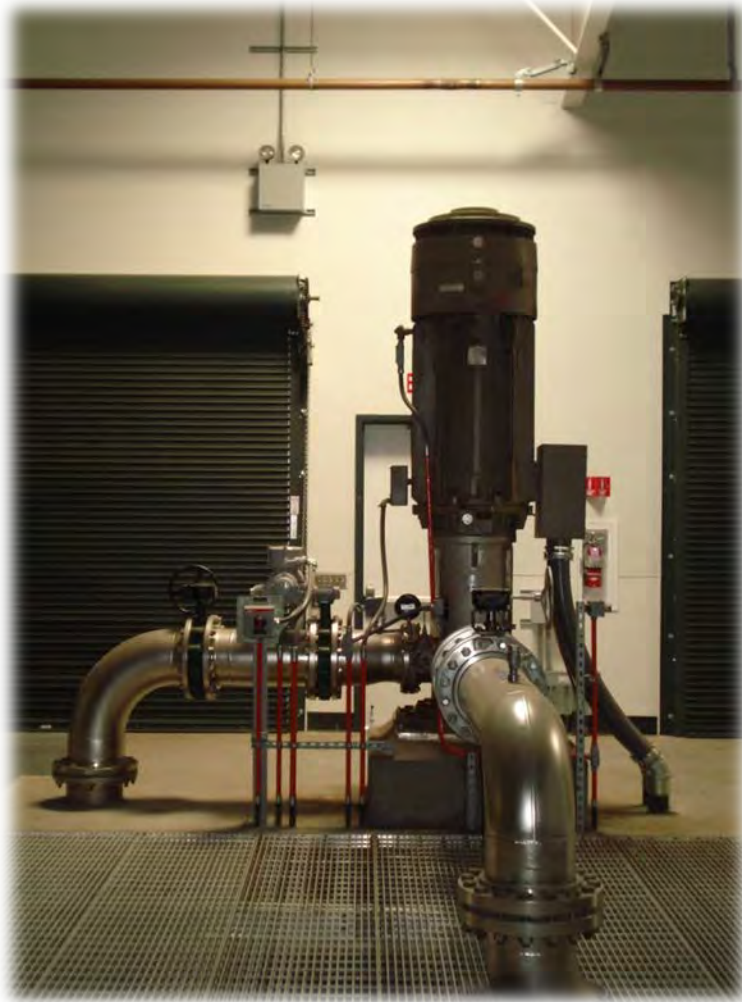
Figure 4.8 RO Feed Pump
