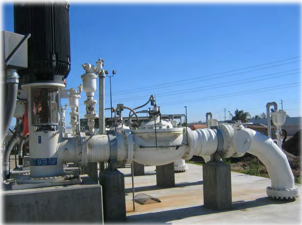
Figure 4.12 Can-Mounted Vertical Turbine Product Water Pump Station
