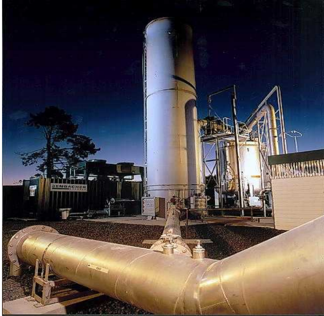
Picture 10. Leachate Evaporation System. Source [7].
