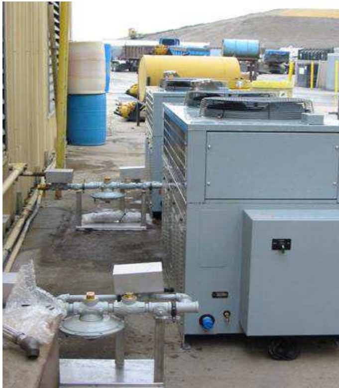
Picture 20. 50 kW installation at a landfill in Michigan. Source: [38]
