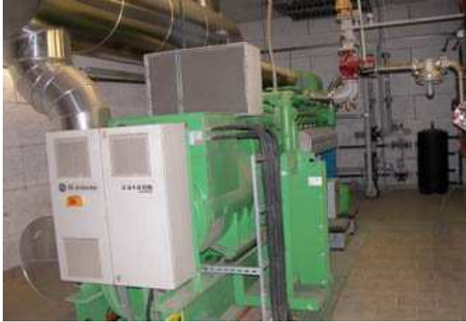
Picture 11. Gas-powered Jenbacher engine with 526 kW power output. Source: [25].
