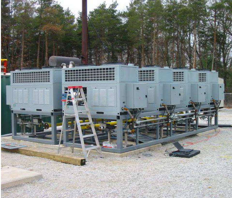
Picture 21. 200 kW installation at a landfill in Michigan. Source: [38]
