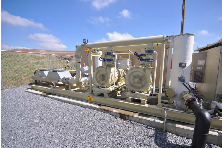
Picture 5. Gas collection system on Oaks landfill, USA.
