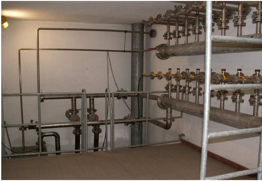
Picture 3. Landfill Gas Collection Station Source: INiG photo.
