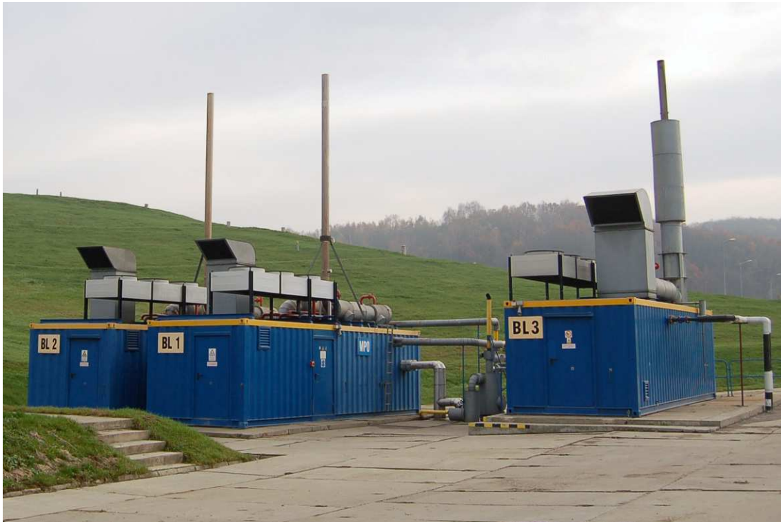
Picture 15. Reciprocating engines enclosed in containers at Barycz landfill. Source: INiG photo.
