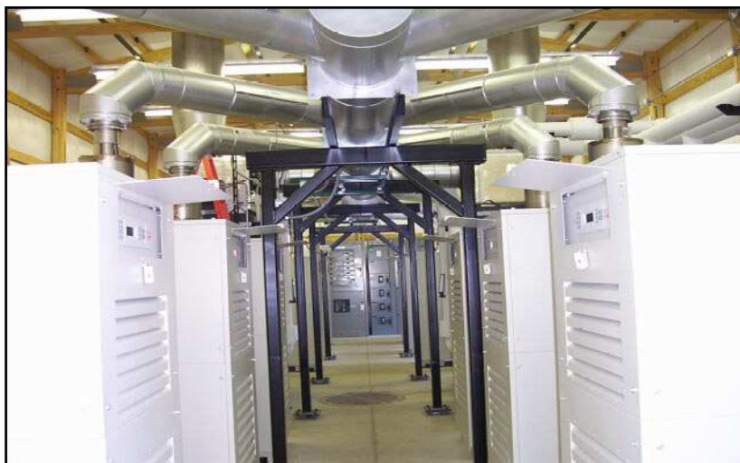
Picture 17. Microturbines in the methane co-cogeneration plant in Antioch Community High School Source: [33]
