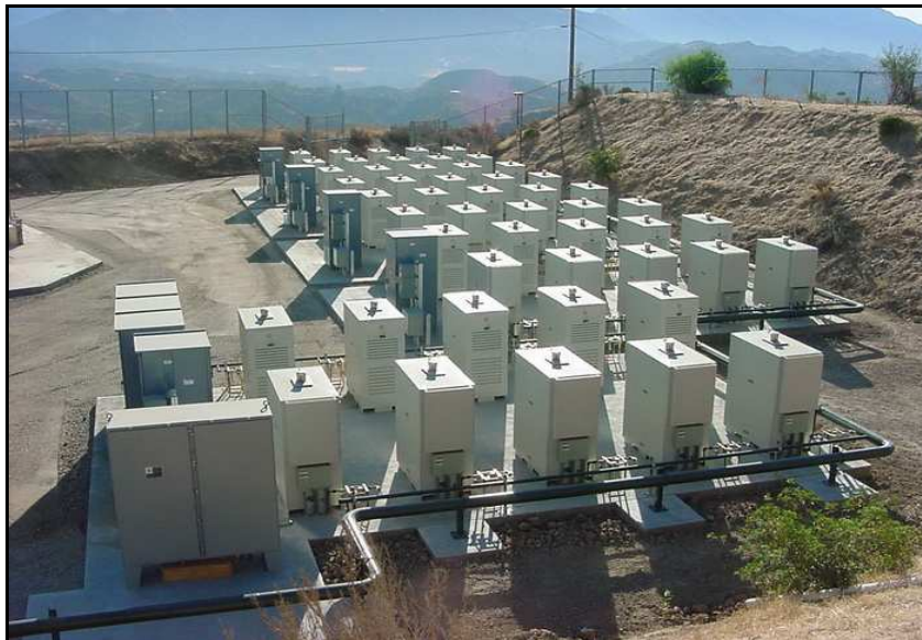
Picture 18. Microturbines at Lopez Canyon Landfill. Source: [36]
