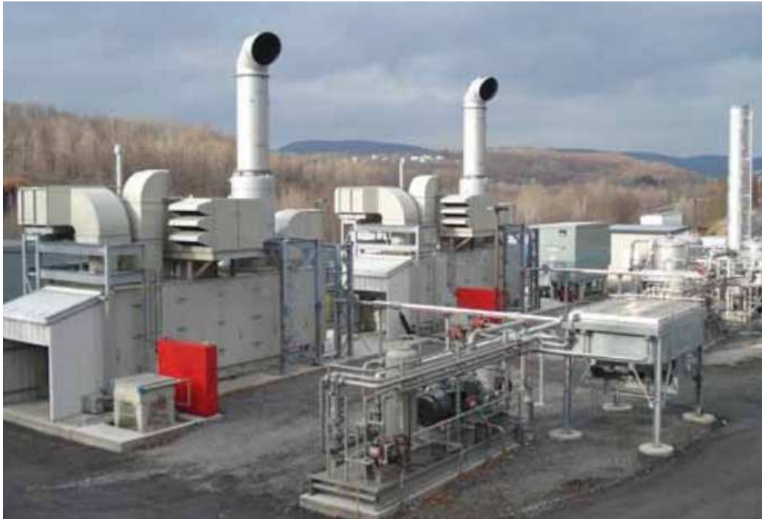
Picture 16. Landfill gas-fueled power facility in Archbald, Pennsylvania. Source: [28].
