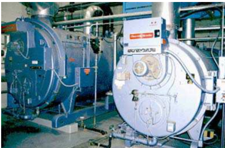
Picture 6. Boiler fuelled by landfill gas. Source: [7].
