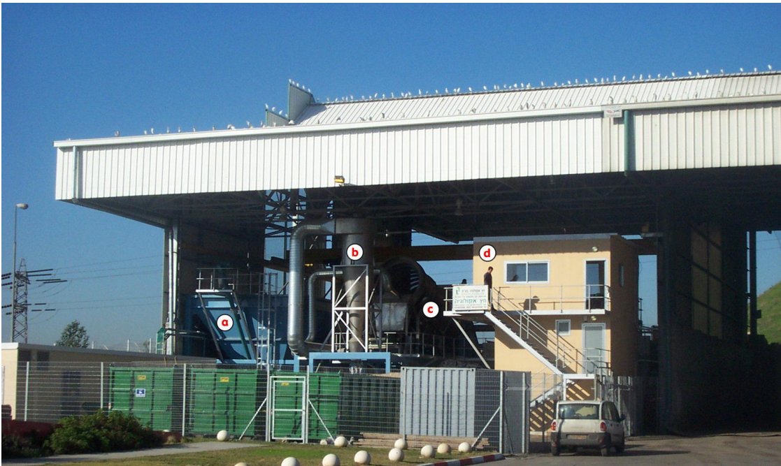
FIGURE 2. VISITOR ENTRANCE TO THE FRONT-END PHYSICAL SEPARATION AND PREPARATION STAGE (BINS IN FOREFRONT REMAIN FROM CONSTRUCTION).
