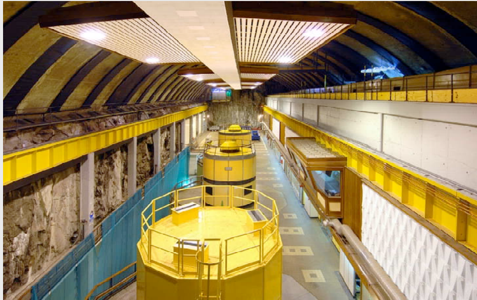
■ The station's machine hall, containing the four turbines, is the same size as a football pitch
