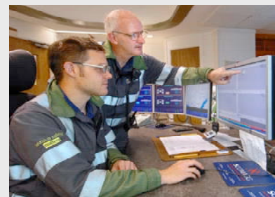
■ Cruachan Power Station control room
