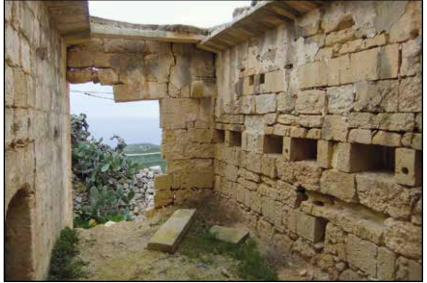
A one-roomed building in Imtahleb devoid of its roof showing the use of kileb
