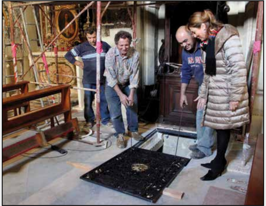
Simone Mizzi with 'Muzzan' father and son, Michael and Patrick Scerri, during the installation of the wrought iron grill over the historic crypt
