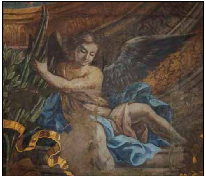
Painting on the vaulted ceiling of Our Lady of Victory Church before and after restoration
