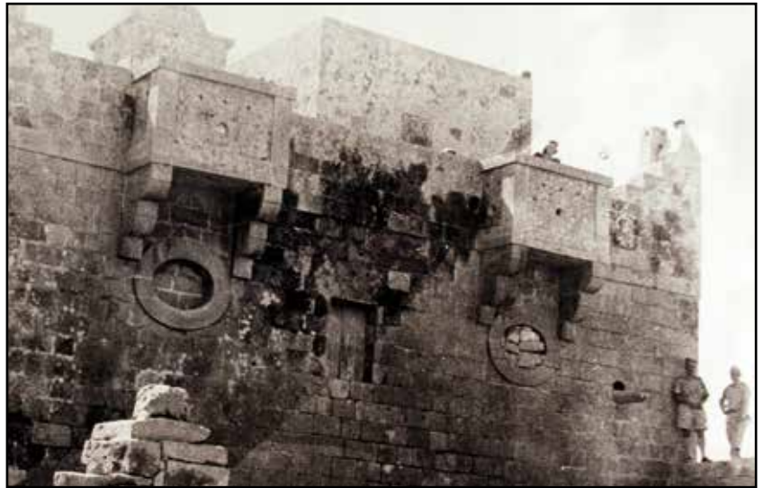
2 of the 8 small balcony-like structures hanging on the upper edge of the first floor level of the west elevation.
