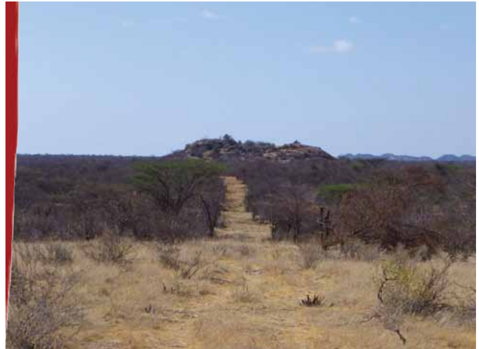
Sera conservancy has carved out a new fence line through the bush for its rhino sanctuary, using local labour.
