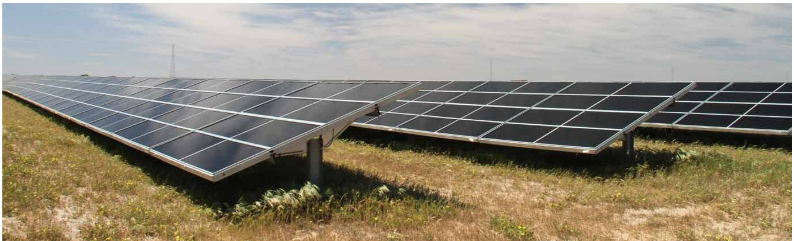
Greenough River Solar Farm, Walkaway
