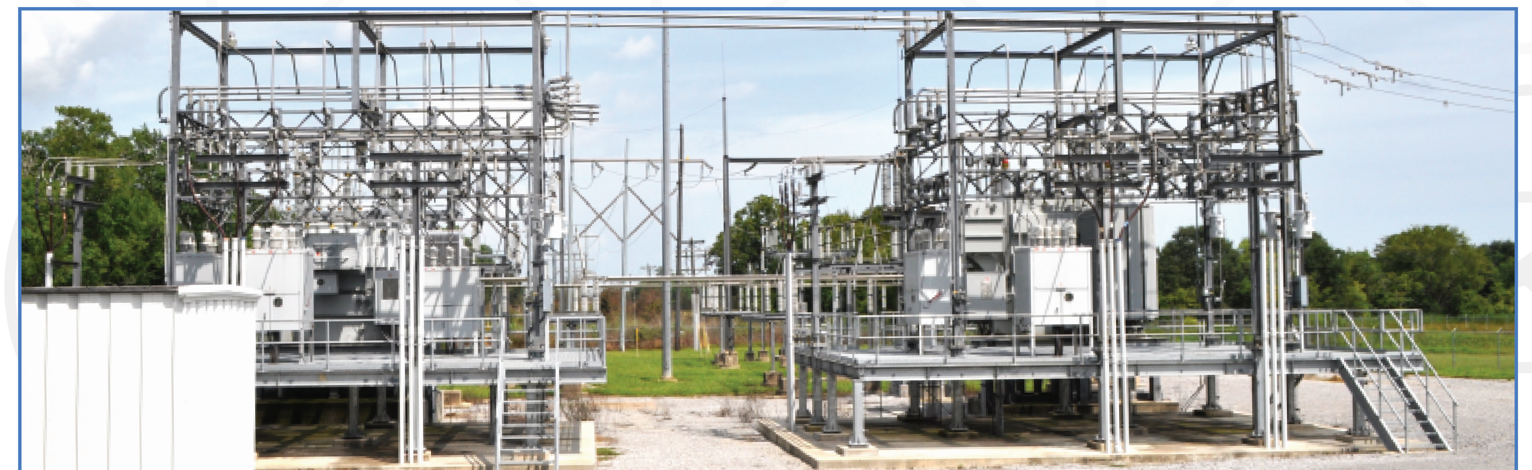
CASE STUDY: 115-24.5KV Outdoor Open-Air Substation
