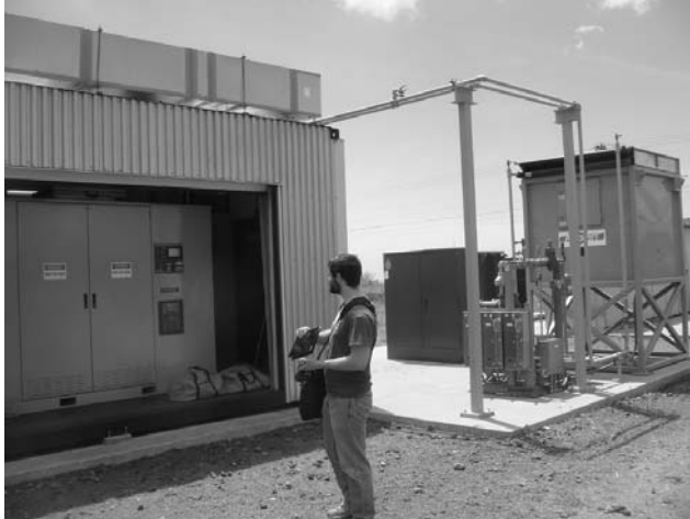
Fig. 1. A grid-connected 1.5 MW-hr lead-acid battery storage system located in Lanai, Hawaii. By convention, at the metering point between the storage system and the grid, power is positive when the grid is charging the battery, and power is negative when the battery (through an electronic inverter) delivers power to the grid. The system rapidly switches between these modes to support fluctuations in power output from an adjacent 2MW photovoltaic array.
