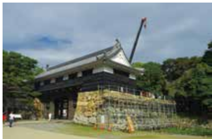
Repair work of stonewall of ruins of Kochi-jo castle (Kochi City, Kochi Pref.)
