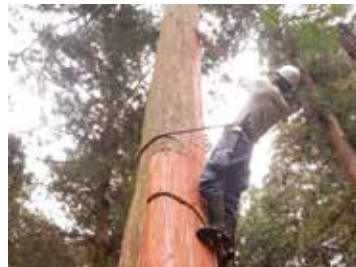
Selected Conservation Techniques: Hiwada Saishu A technique of removing cypress barks which is required for preservation of building with cypress covered roof
