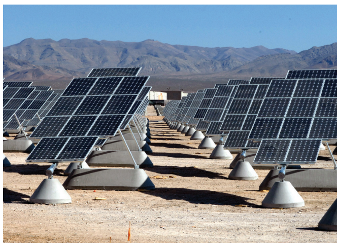
Nellis Solar Power Plant at Nellis Air Force Base in the U.S. The panels track the sun in one axis.
