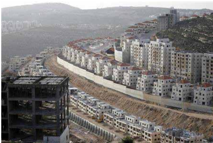
Building a Palestinian nation: houses and apartment buildings under construction in Ramallah, 2012
