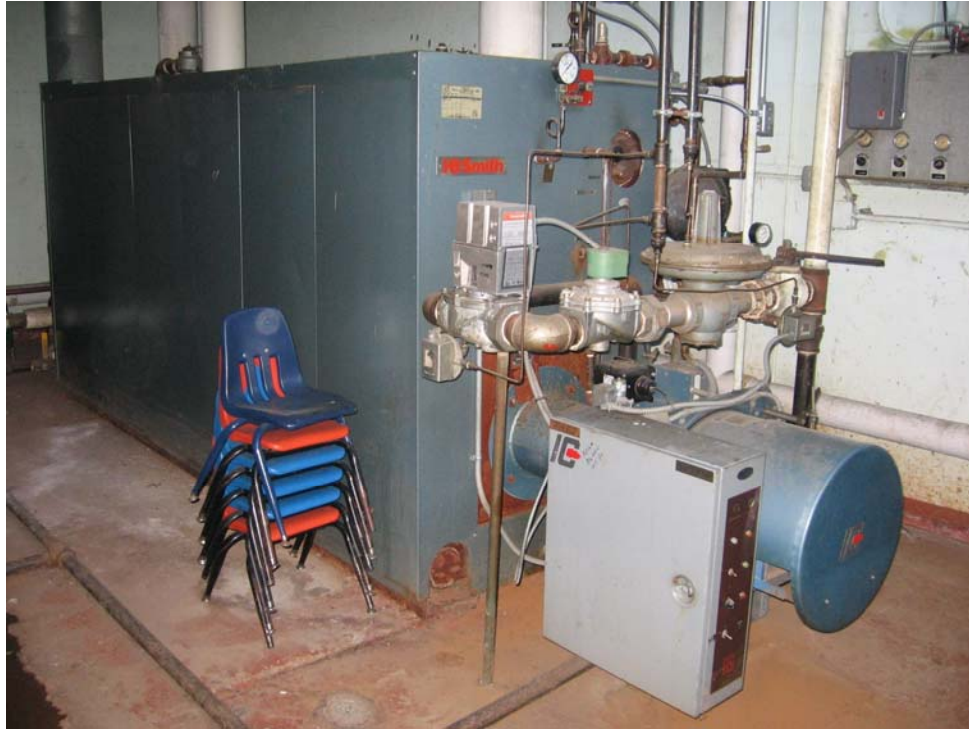
1989 SECTIONAL BOILER AT DONAHUE SCHOOL; NOTE PNEUMATIC CONTROLS ON WALL
