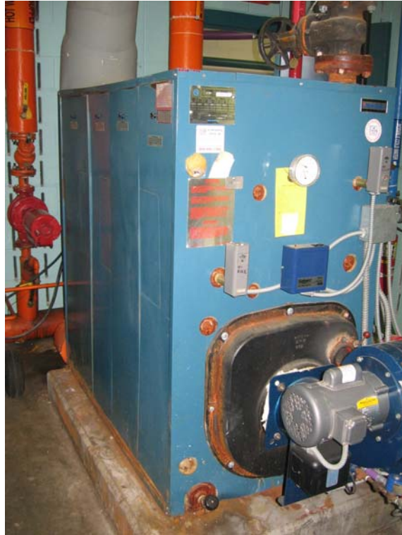
WATER TREATMENT PLANT BOILER RUNS YEAR-ROUND
