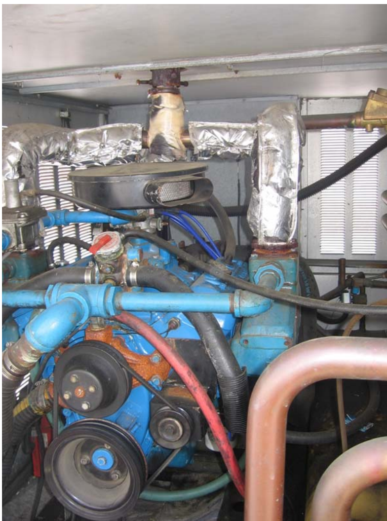
CLOSE-UP OF INEFFICIENT GAS-FIRED ENGINE DRIVING CHILLER AT HG&E HEADQUARTERS
