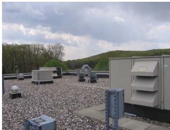
WATER TREATMENT PLANT ROOFTOP UNIT PROVIDES NON-STOP COOLING AND REHEATING TO SILO ROOM
