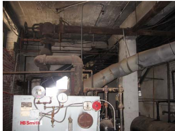
NO STEAM PIPE INSULATION [CITY HALL ANNEX]
