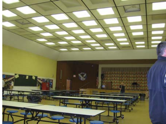
INEFFICIENT LIGHTING IN KELLY SCHOOL CAFETORIUM
