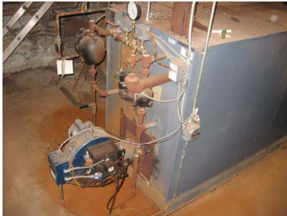
OLDER OIL-FIRED CAST IRON BOILER IN HOLYOKE CITY HALL
