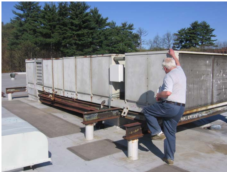
FAILING ROOFTOP UNIT AT PECK SCHOOL
