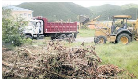
A backhoe (right) dumps debris into a dump truck (right) during the cleanup of the Belvedere neighbourhood on Sunday.
