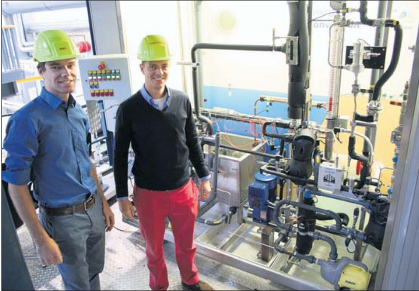
Bluerise Chief Technical Officer and co-founder Ir. Berend Jan Kleute (left) and Bluerise Vice-President Engineering Ir. Joost Kirkenier at the OTEC installation at Technical University Delft Process and Energy Lab.
